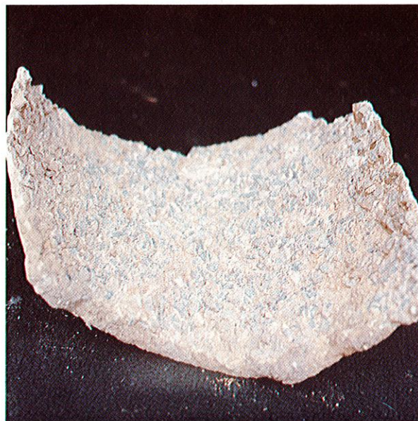
Remainder of bottom third of 225 mm O-G jointed concrete pipe from a sewer downstream of a pumping main discharge which had failed after less than 10 years service. The aggregate exposed after the cement had been attacked by sulphuric acid oxidised from atmospheric hydrogen sulphide in the presence of moisture is clearly visible.
