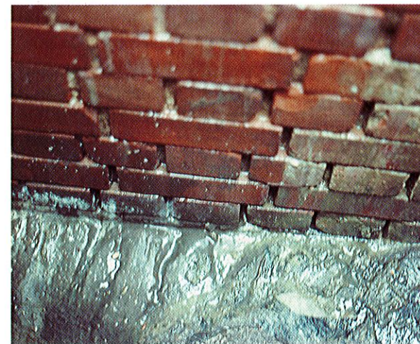
Attack by sulphuric acid oxidised from atmospheric hydrogen sulphide in the presence of moisture at a pressure main outfall. Most of the mortar between the clay bricks has disappeared and the concrete benching has been severely attacked.
