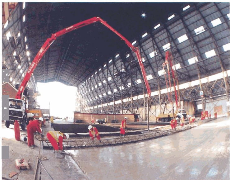
Figure 1 This 500 m 3 concrete strong floor at BRE's Cardington laboratory used 100 tonnes of Class RCA(III) coarse aggregate
